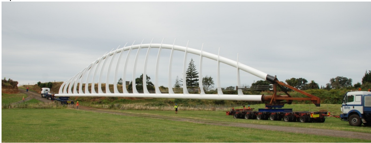
Figure 3: The Te Rewa Rewa Bridge superstructure being transported to site from the fabrication workshop. The superstructure as shown was approximately 85m long and weighed 85 tonnes. The journey distance was 1.5km across mainly unpaved tracks.
